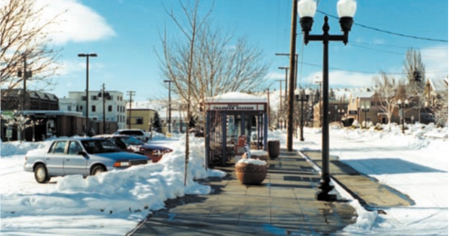
In Klamath Falls, Oregon, a geothermal district-heating system keeps the sidewalks clear and dry at the Basin Transit station after a snowfall.
