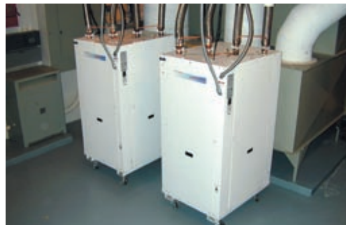
Two 36-ton heat pumps being used for space heating at the College of Southern Idaho.
