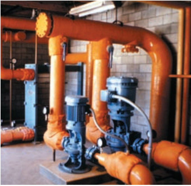
Heat exchangers and circulation pumps for the geothermal district-heating system in Klamath Falls, Oregon.
