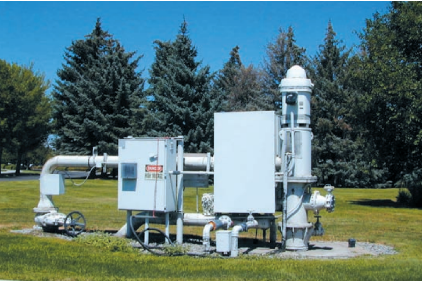
Geothermal production well at the College of Southern Idaho, Twin Falls. This district-heating system now heats nearly half a million square feet (46,450 square meters), with more area reached by this winter with 16 heat-pump units.
